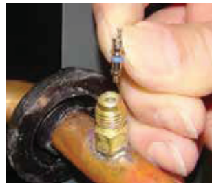
A. Remove the valve stem from the Schrader port mounted on the suction line.
